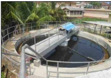
Figure 3 - Sewerage plant at Teaching Hospital Batticaloa
